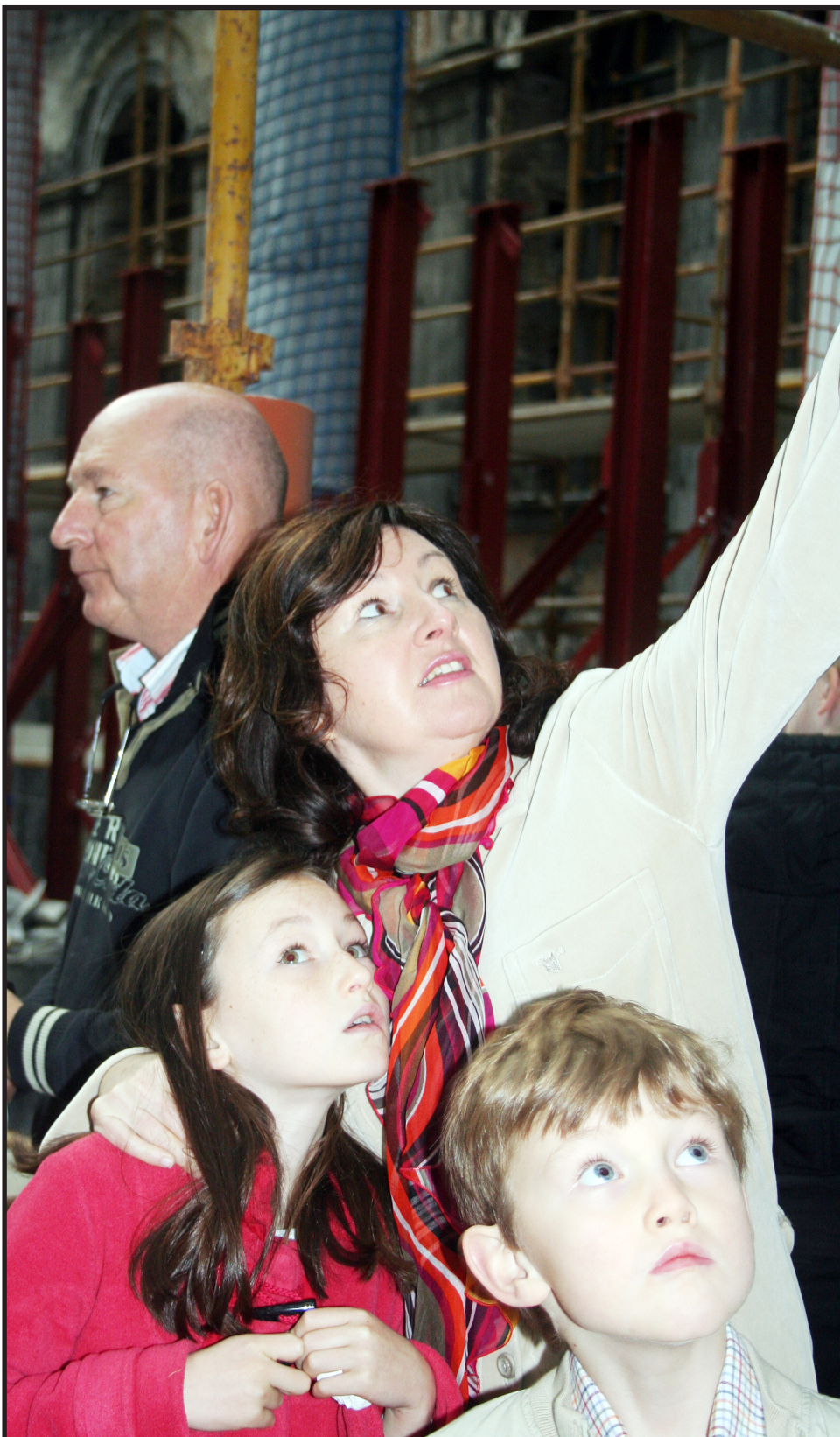
Some of the keen visitors view the fire damage at St. Mel's Cathedral.
